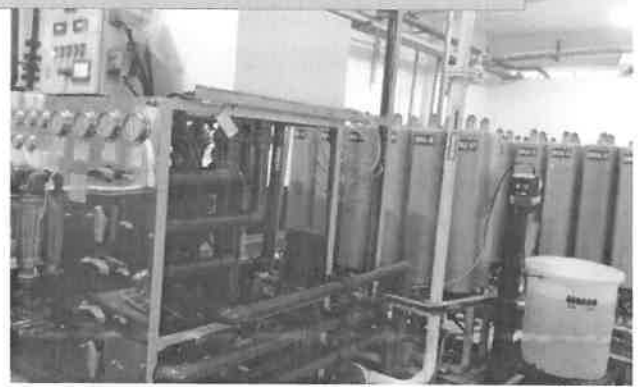
Reverse Osmosis (RO) system
