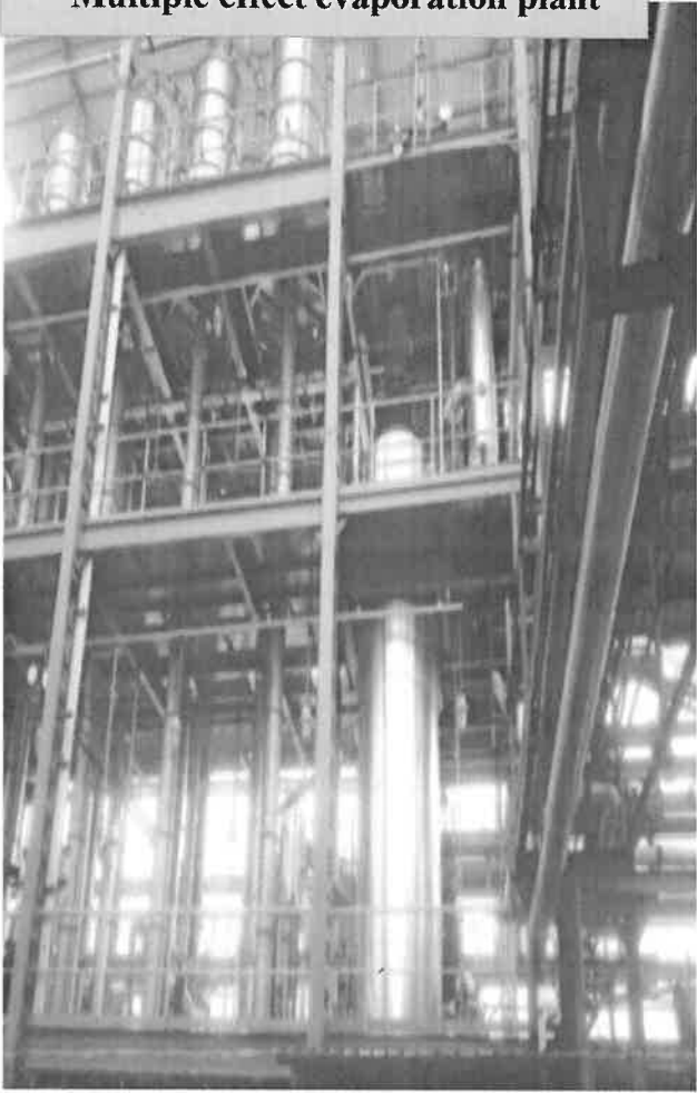
Multiple effect evaporation plant
